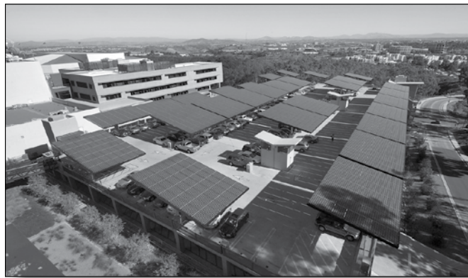
Solar Trees on Hopkins parking structure
